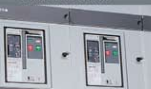
POWER DISTRIBUTION & CIRCUIT PROTECTION
