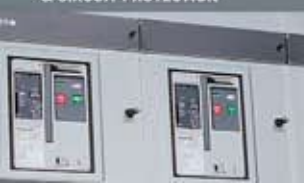
POWER DISTRIBUTION & CIRCUIT PROTECTION
